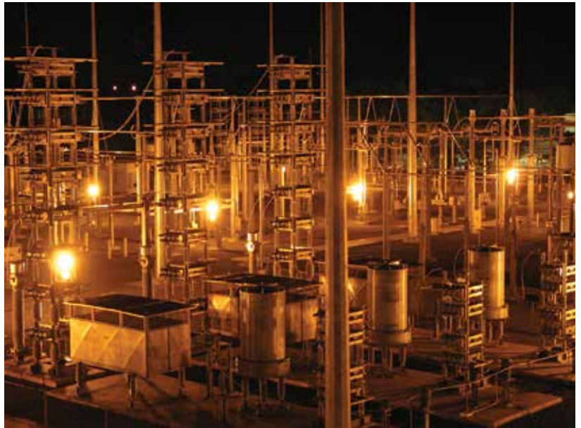
The switchyard at the Neptune Regional Transmission System converter station on Long Island receives direct-current power from the PJM network in New Jersey before converting it to alternating current for use by PSE&G's Long Island customers.
