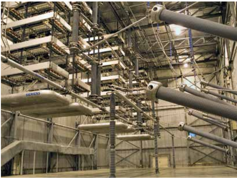
Thyristors convert up to 660 MW of energy from direct current to alternating current inside the valve hall at Neptune Regional Transmission System's Duffy Avenue converter station. Since commercial operation began in 2007, Neptune has provided approximately 20% of the electric power used on Long Island.
